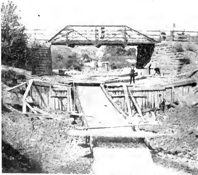
Fig. 1—Crichton Road bridge, showing washout and contractor's chute.
